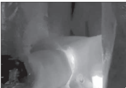
Leak in a 4-way valve dryer skid
