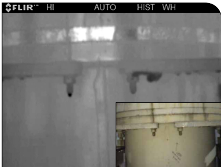
Visible vs. OGI image of SF 6 leak
