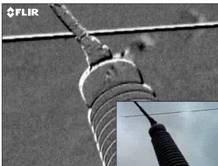
SF 6 leaking from the bushing of a gas circuit breaker
