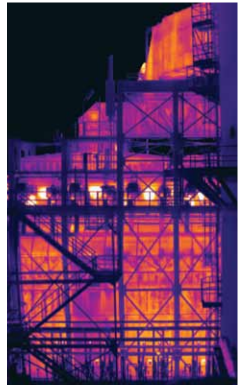
A cabin furnace as seen from a distance of about 80 meters using the FLIR P640 thermal imaging camera.
