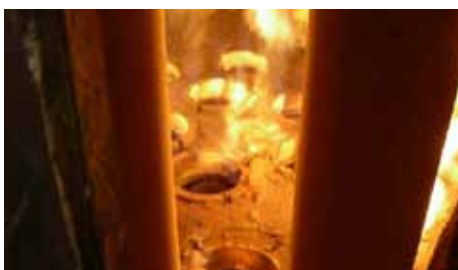
Inspection ports provide a view of internal parts, but flames, combustion gases, and ash obscure the equipment during operation. A FLIR thermal imaging cameras with a flame filter is not hindered by such obscurants.
